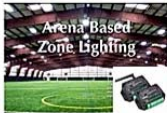
Zone lighting to deactivate unused lights to save energy
